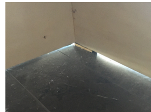
4. Bottom of recess not sealed, allowing air leakage.
