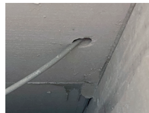
2. Cable penetration not sealed.
