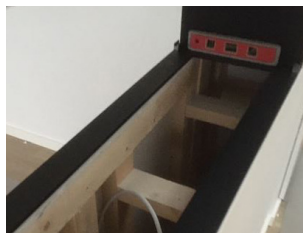
1. Combustible material inside recess (not permitted).
