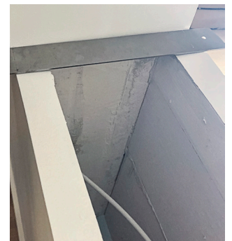
The 2 wall must be in level.
