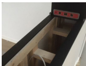
1. Combustible material inside recess (not permitted).
