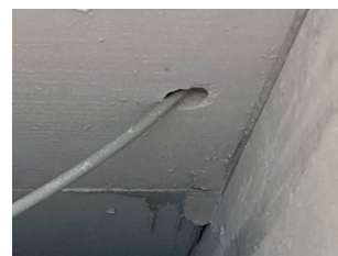
2. Cable penetration not sealed.
